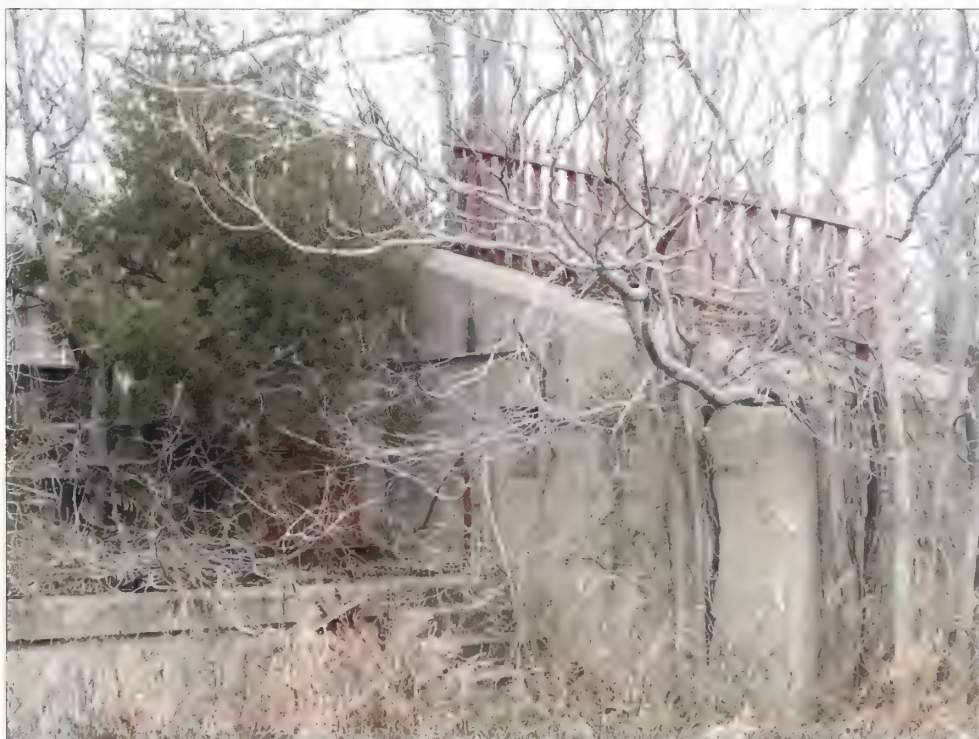
Figure 5.34. Wood picket fence on top of Battery Morris. The entire length of the pictured non-historic fence should be removed. Great care should be exercised not to damage the historic concrete structures and the historic earthwork north of the battery when the posts are removed (Olmsted Center, January 2009).
